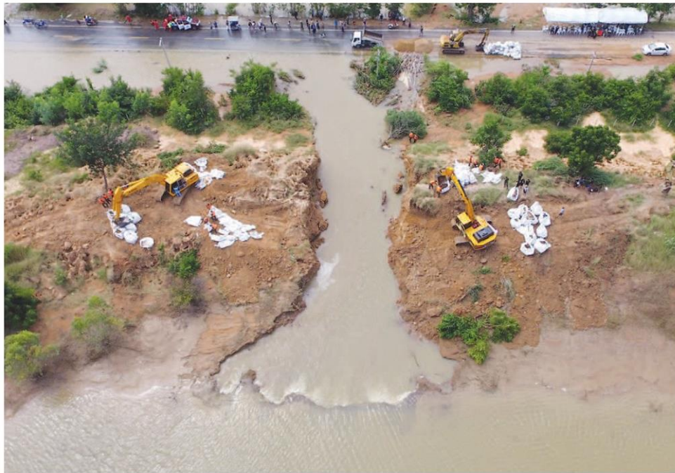
This aerial picture shows the site of breached earth dam in Lop Buri, which has caused widespread flooding in nearby farmland and villages.
